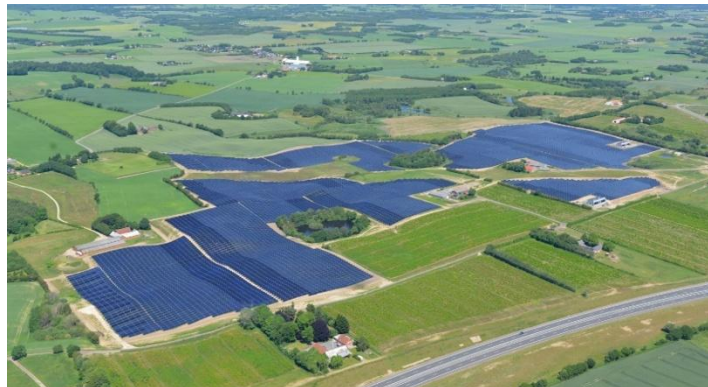
World's largest solar thermal system at Arcon-Sunmark in Silkeborg/Denmark © GREENoneTEC
